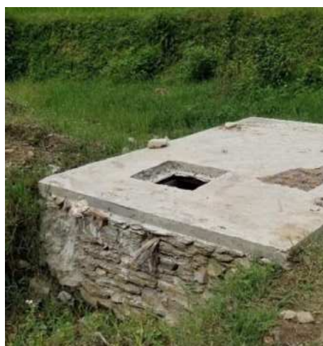
Figure 9: Example of water source protection
